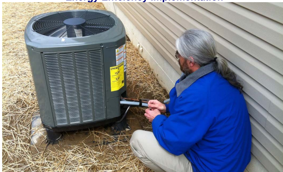
Figure 5: High-Efficiency Air-Conditioning Unit as an Example of Energy Efficiency Implementation
