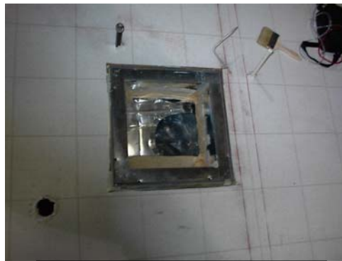
Furnace plate sealed with mastic.
