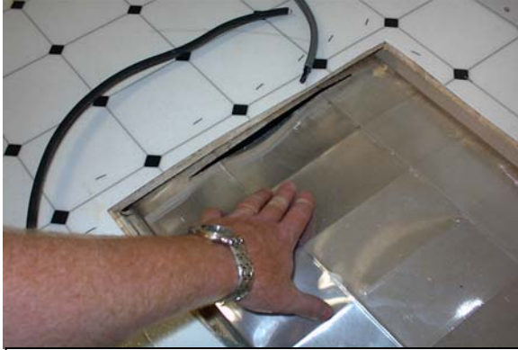
Branch ducts have zero clearance for saw cut through floor sheathing; the picture frame cut cannot be used.
