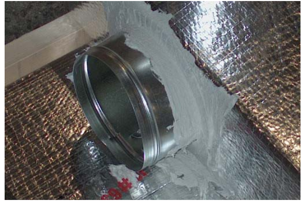
Applying tape as a temporary seal then covering the seam and tape with mastic will result in a superior and durable seal.
