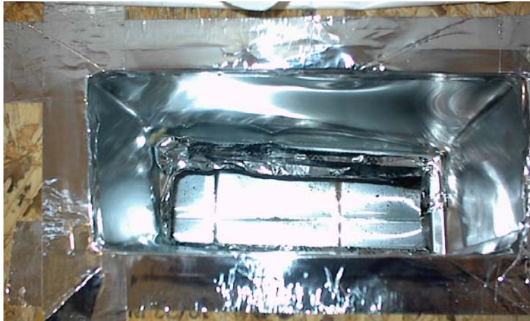
In-line supply connector showing tape at trunk connection. Cutting a properly sized hole and applying mastic to the connector prior to insertion into the floor is the preferred method of insuring a good seal.
