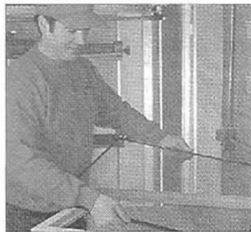
WINDOW SASH IS REMOVED AND MODIFIED TO RECEIVE INSULATING GLASS UNIT, EXISTING MUNTINS APPLIED TO SURFACE
