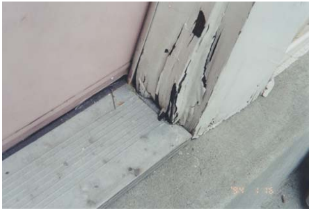
Figure 26 Rot at the bottom of a door frame in a 1990s sample house.
