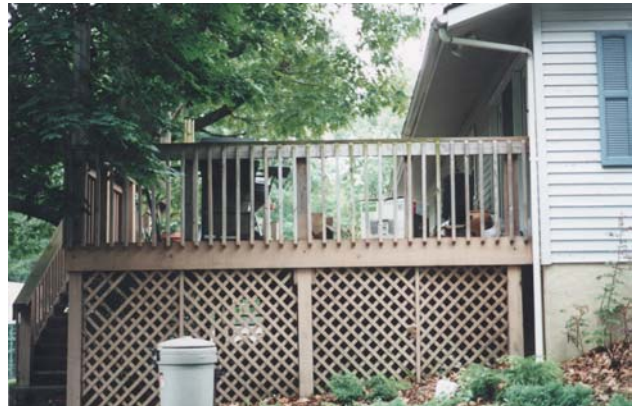
Figure 55 Example of a wood deck in good condition (1970s house sample; age of deck unknown).
