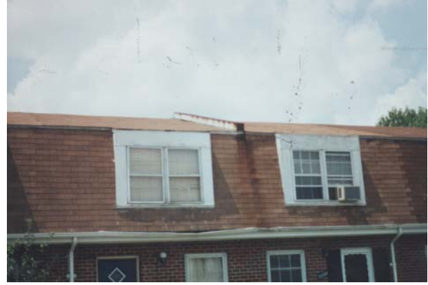
Figure 45 Rusting party wall cap flashing and damaged gutters.
