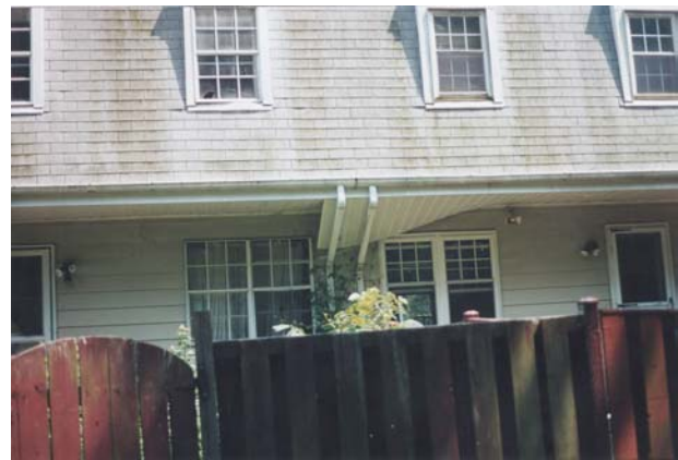
Figure 33 Broken window pane on second-story window.
