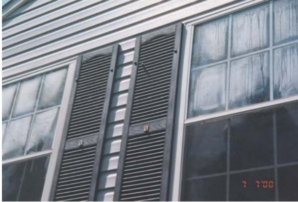
Figure 34 Condensation inside double-pane windows.
