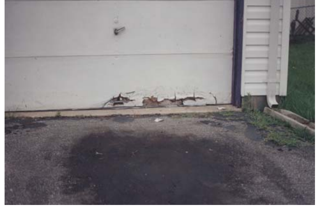
Figure 31 Rot of wood composite panel on a garage door (1970s house sample).
