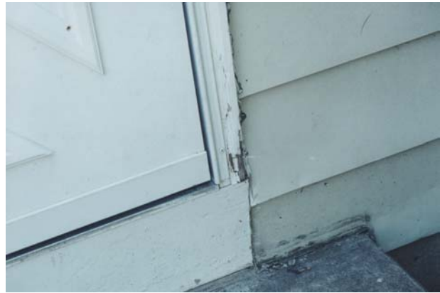
Figure 27 Rot at the bottom of a door frame and trim in a 1970s sample house.
