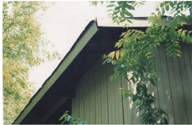
Figure 37 1970s sample house with wood fascia needing minor repair (rated adequate by inspector).
