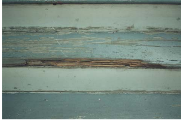
Figure 53 Wood floor boards under the porch roof of a 1990s house sample show signs of deterioration.
