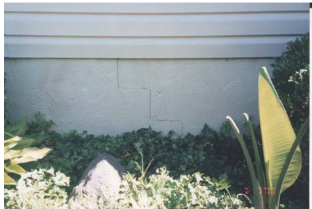
Figure 25 A typical small crack found in a masonry foundation wall.
