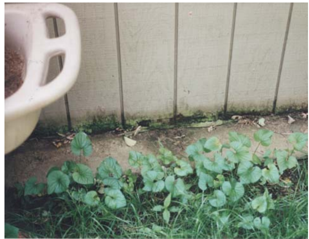
Figure 29 Rot at the bottom of wood panel siding (insufficient ground clearance) in a 1970s sample home.
