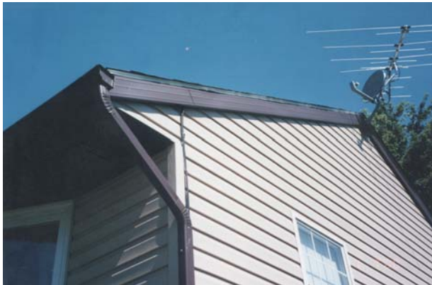
Figure 36 Example of aluminum fascia covering older fascia material on a 1970s sample house (rated good by inspector).
