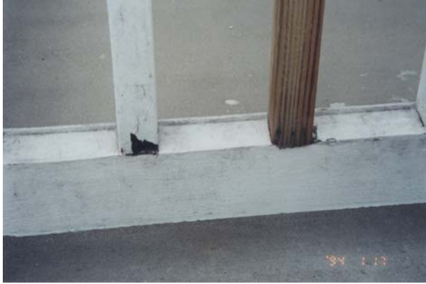
Figure 52 Rot in a wood picket on the porch of a 1970s sample home (one picket has been replaced with treated wood).
