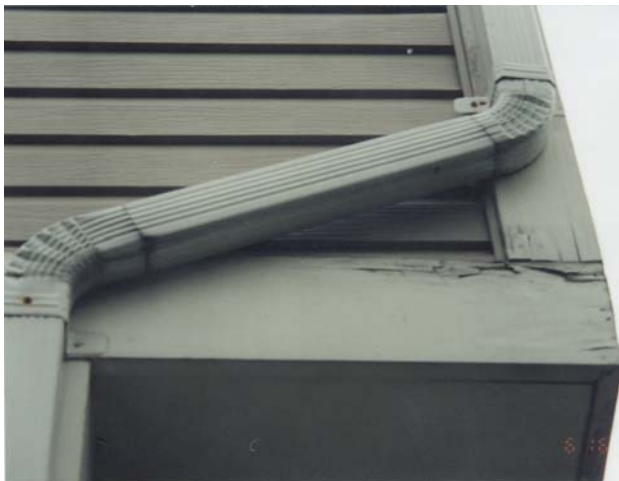
Figure 28 Rot in exterior wood trim of a 1990s sample house.
