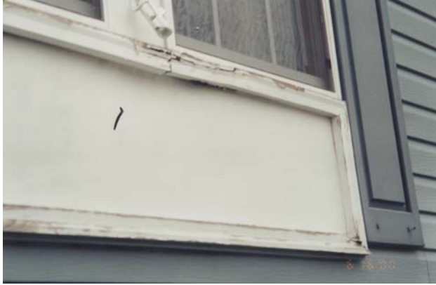
Figure 30 Rot in wood trim associated with poor detailing (i.e., lack of cap flashing) and maintenance in a 1990s sample home.
