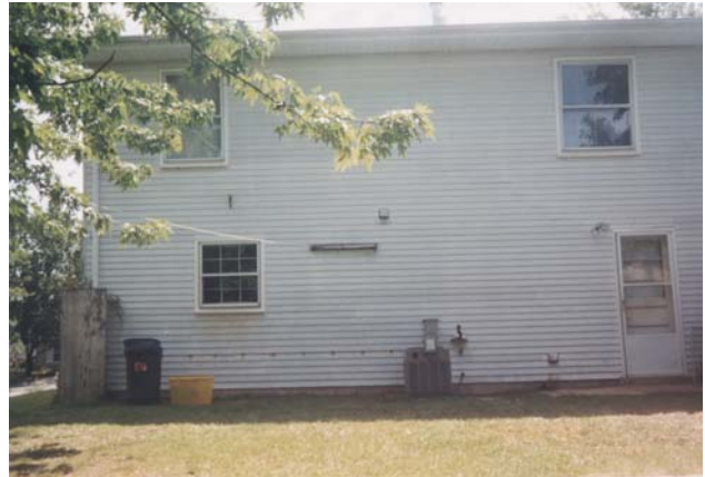
Figure 23 Example of poor rating for site grade and drainage.
