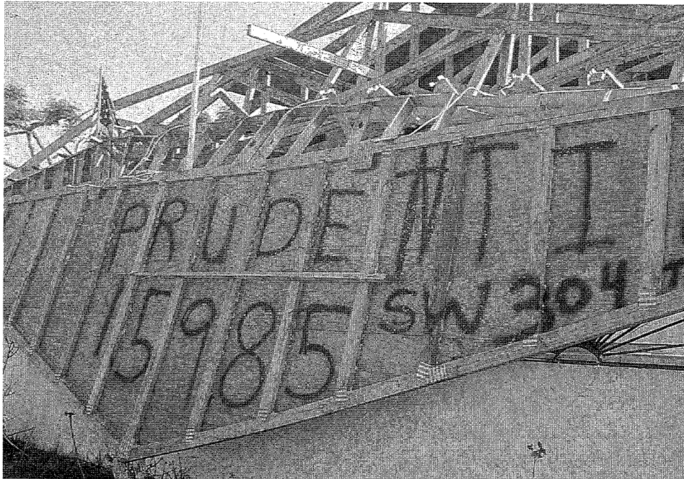
Figure 22. A gable-end truss dangling by hurricane straps.
