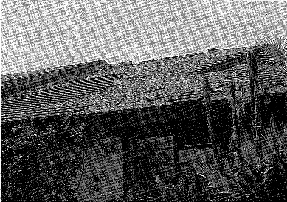
Figure 33. Wind damage to a flat tile roof. In part, the use of insufficient beds of cement mortar contributed to this unusual level of damage for flat tile roofing. Roofing underlayment prevented serious water damage. The "Roof" damage rating includes all elements of structural integrity along with water resistance.
