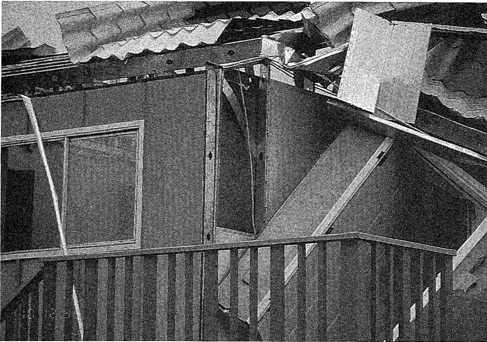
Figure 84. Light-gauge steel framing was also subject to severe damage.
