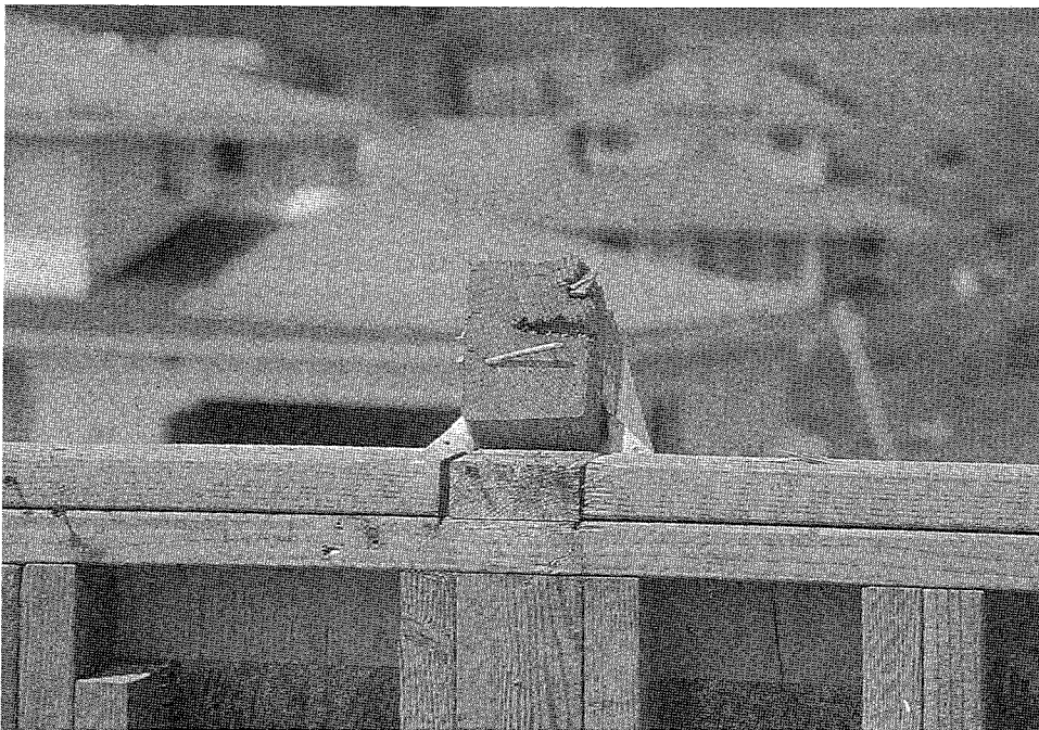
Figure 85. The metal strapping between the first and second story on this home did not provide adequate structural continuity between stories.
