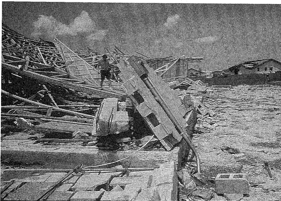
Figure 27. Wind damage to a CBS wall under construction. Note the rebar withdrawal at the corner of the concrete tie beam and the absence of rebar for the wall in the foreground.
