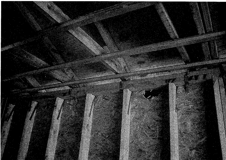
Figure 48. Resilient steel channels used behind drywall render the ceiling diaphragm less effective by detaching the drywall from the roof trusses.
