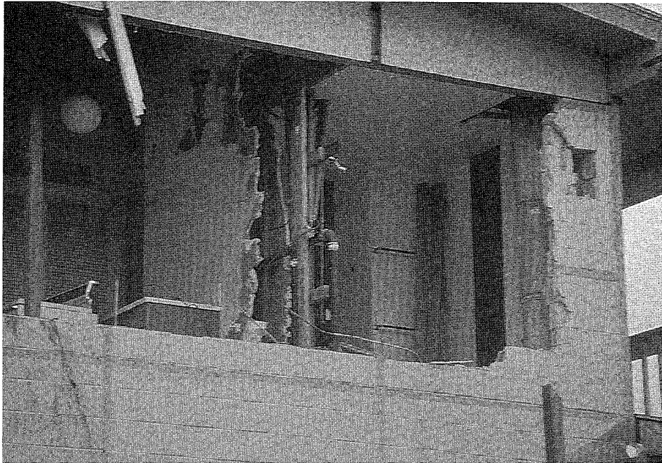
Figure 82. Blown out concrete block end wall that lacked a concrete tie beam and proper reinforcing.
