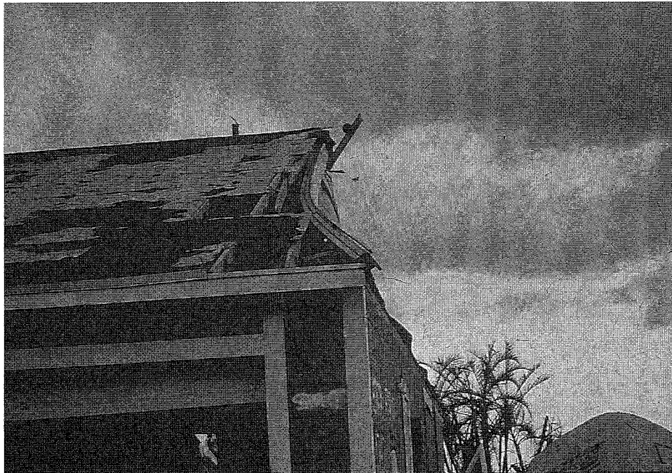
Figure 19. Wind damaged gable end wall. This home was not part of the random sample.
