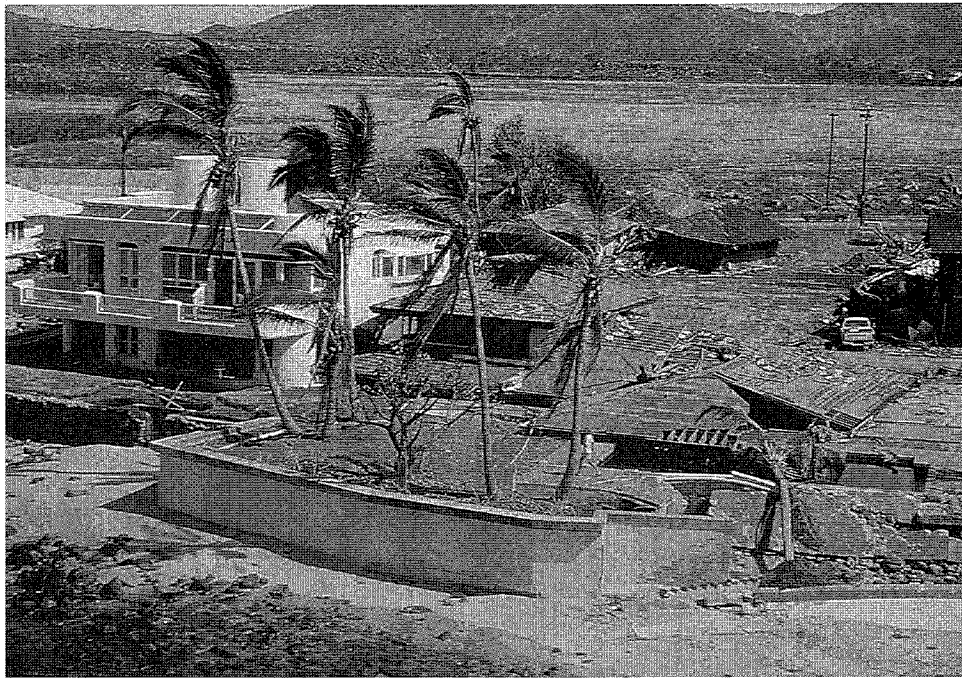
Figure 109. Storm surge damage to adjacent unelevated homes. The home on the left allowed the storm surge to pass through the lower level, which reduced the surge pressure on the structure.
