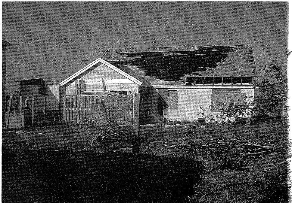
Figure 35. Wind damage to a composition shingle roof. Composition shingles were almost completely removed on many homes by Andrew's winds. The extensive water damage overrides the relatively sound structural condition of this house.
