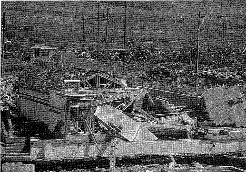
Figure 94. Slab-on-grade foundation survives the storm surge but the remainder of the home was demolished by storm surge. Away from the coastal flood plain, slab-on-grade foundations performed well.
