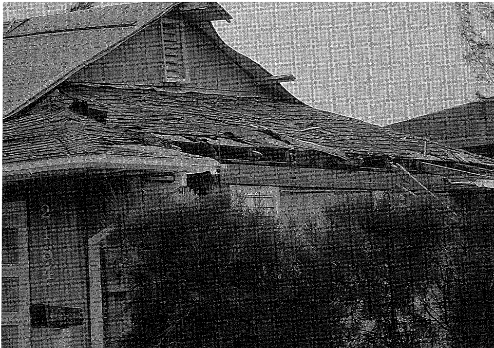
Figure 71. Roof framing at overhangs was particularly vulnerable.
