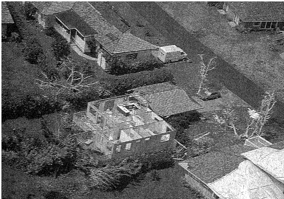
Figure 73. This home lacked a continuous load path from the roof to the walls and lost its entire roof.
