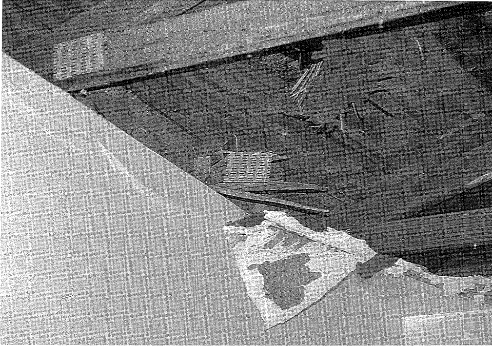
Figure 104. A wood projectile penetrates roof framing materials.
