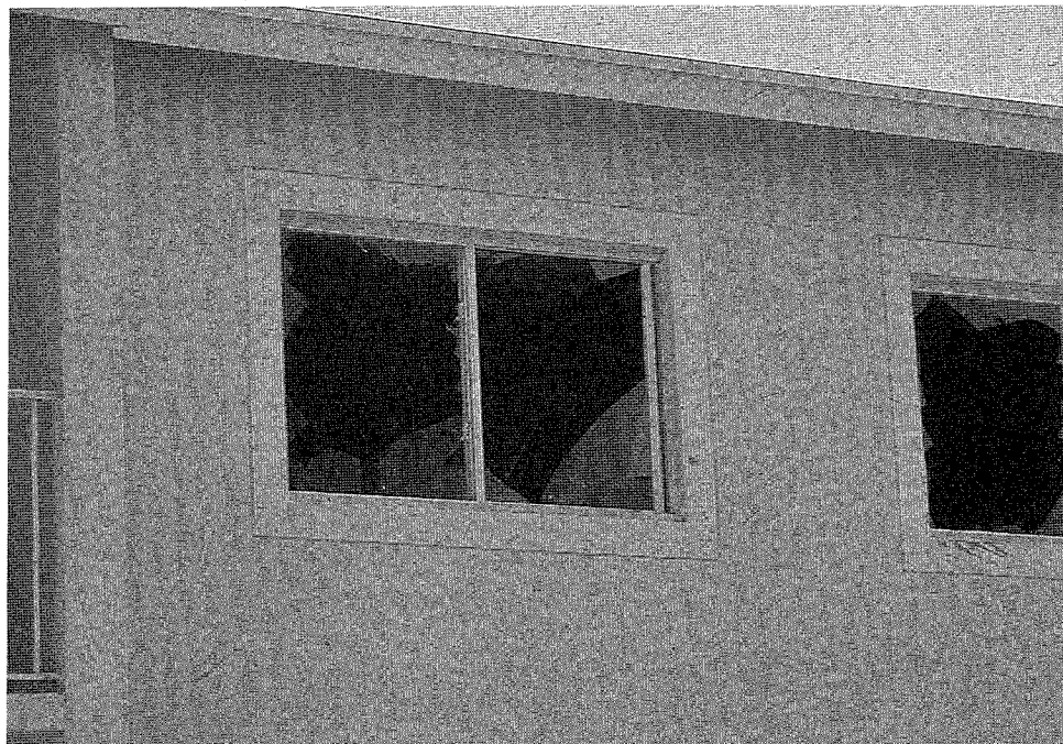
Figure 38. Illustration of damage to unprotected windows.
