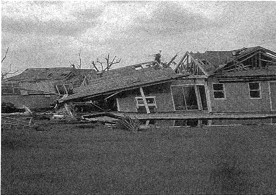
Figure 44. Complete failure of a wood framing system: shattered windows, failed porch overhang, detached roof sheathing, collapsed gable end, and fallen drywall ceiling. Exterior walls are severely racked from reduced lateral support from the tattered roof structure and inadequate shear wall construction.
