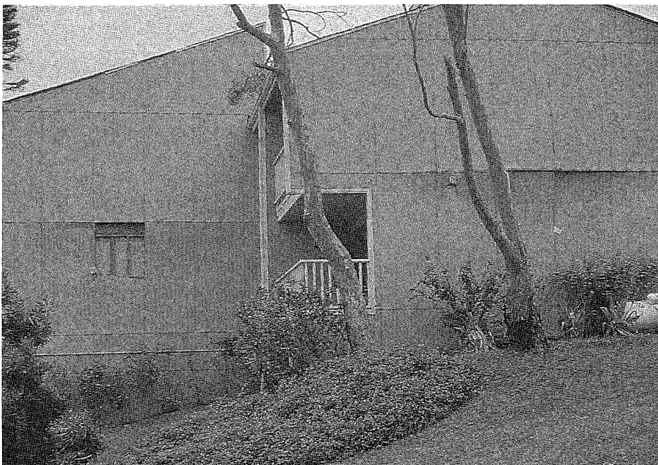
Figure 83. Wood-frame end wall with buckling and tearing of hardboard siding panels.
