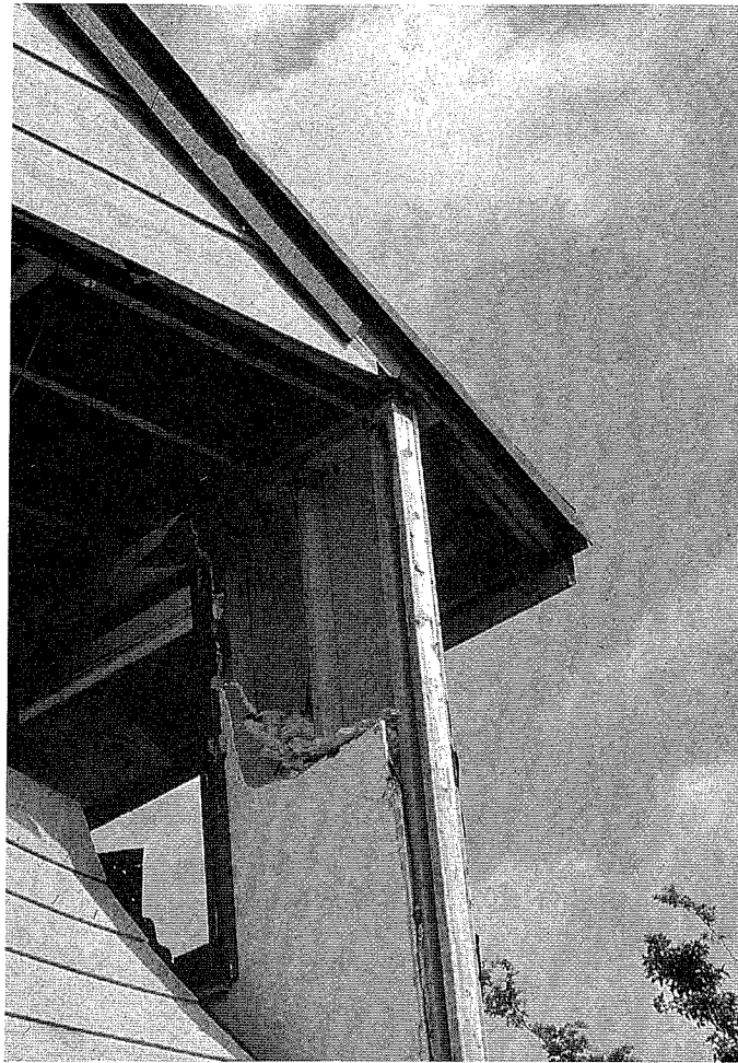
Figure 28. Wind damage to a wood-frame wall (two-story) showing improperly connected corner.
