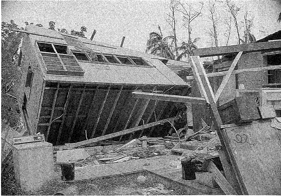
Figure 93. This single-wall home lacked continuous load paths to the foundation and failed by overturning.
