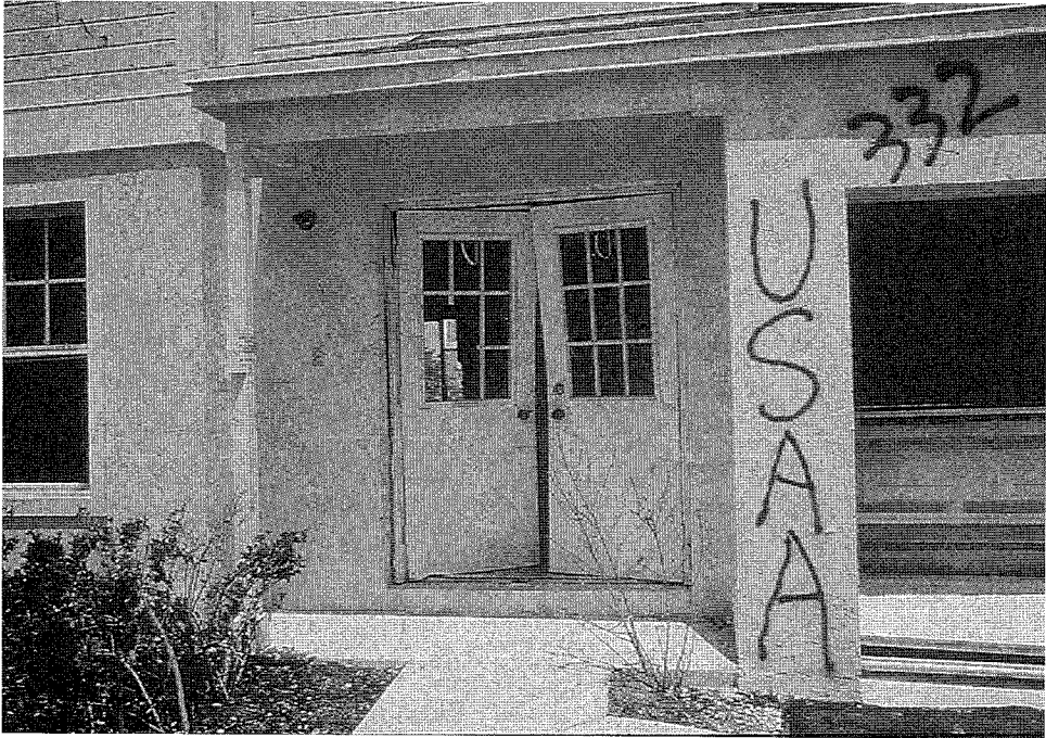
Figure 40. Illustration of damage to double entrance doors.
