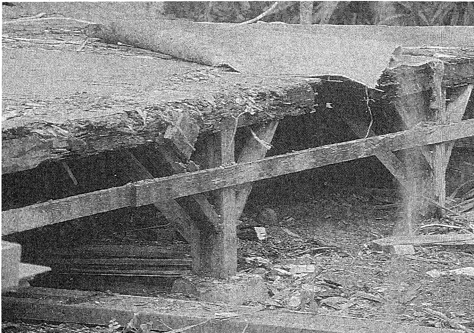
Figure 90. Wood post foundation with severe rot and termite damage.
