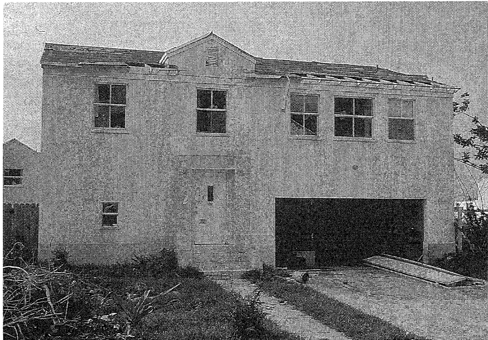
Figure 15. Example of a two-story, wind-damaged house (concrete block). It was noted that all windows were broken and that sheathing was lost from the roof perimeter. The gable ends did not collapse, but the water damage was substantial due to stripped shingles, broken windows, and lost sheathing.
