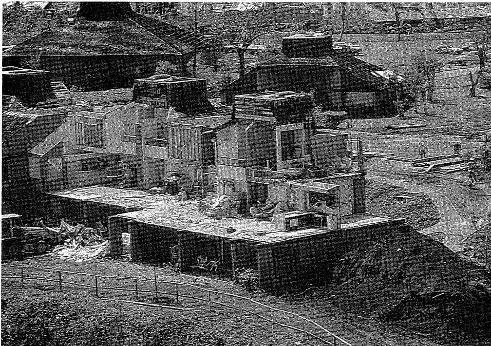
Figure 108. The residences at the top edge of the slope suffered severe damage while those further back were still intact.
