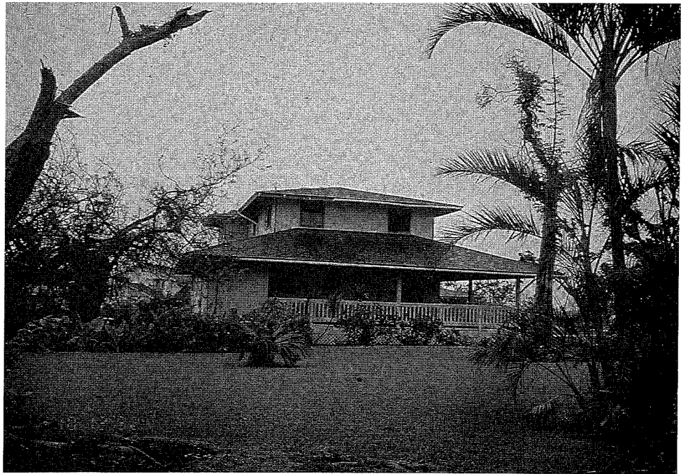
Figure 62. Wind-damaged home with a Level 1 damage rating for overall building condition. This two-story home was built using conventional wood framing with T1-11 siding. The roof is hip shaped with large overhangs and porches. The survival of this home was noted as "excellent," but minor water damage and damaged rain gutters were recorded on the survey form.
