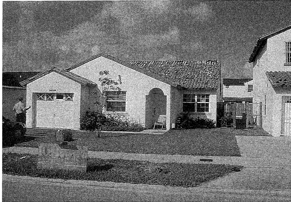
Figure 34. Wind damage to a barrel clay tile roof. In part, the use of insufficient beds of cement mortar contributed to this level of damage for some barrel-clay tile roofing. Roofing underlayment normally prevented serious water damage.
