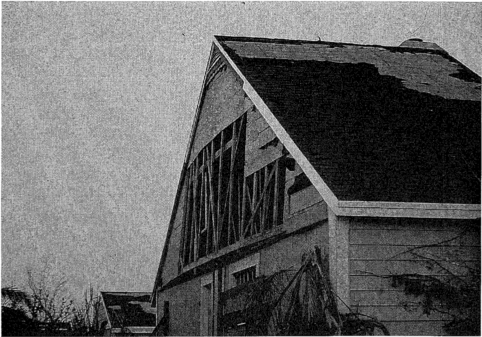
Figure 45. Sheathing blown-out at a gable end wall with a steep pitched roof.
