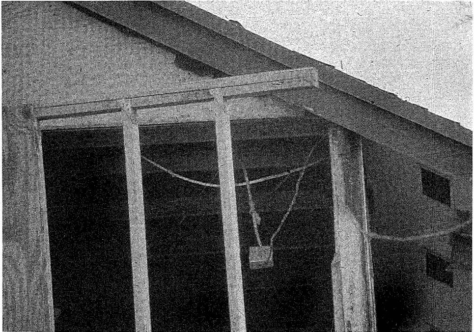
Figure 46. Improper connection of a corner in a blown-out wall section.
