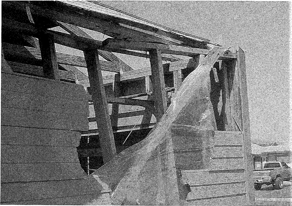
Figure 47. Failure of hardboard exterior wall siding with a let-in brace.
