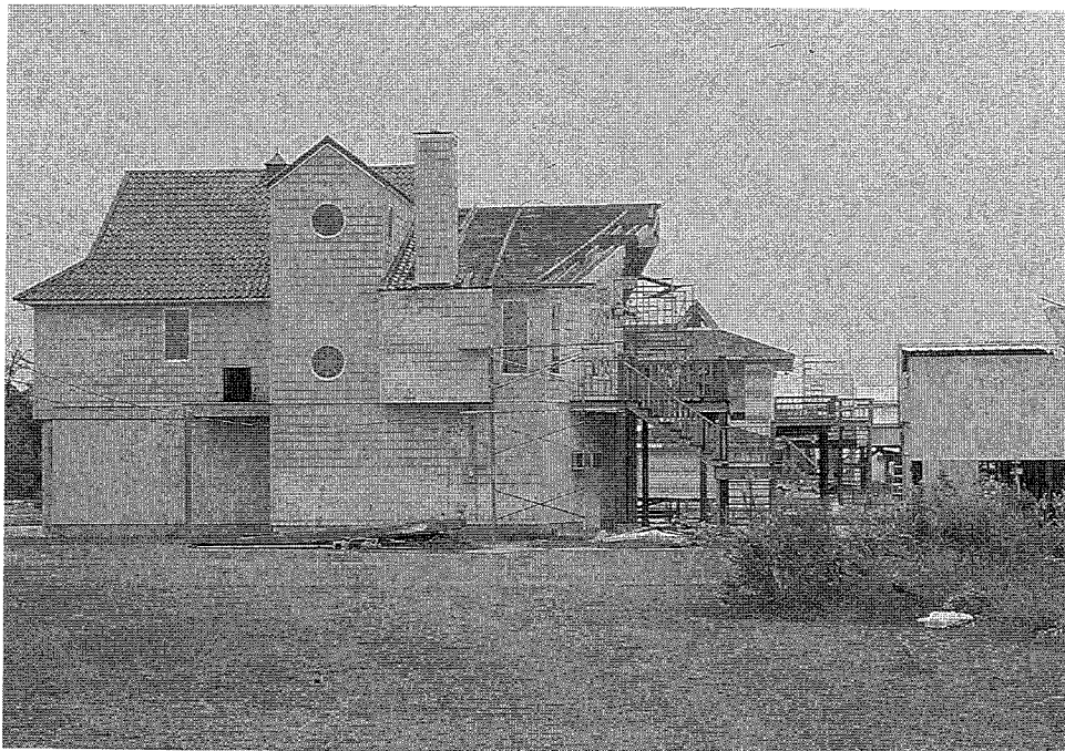
Figure 58. Gable ends and overhangs presented some problems in Louisiana, similar to Florida.
