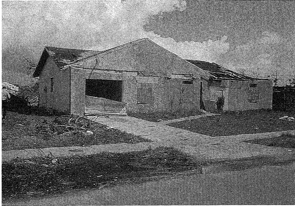
Figure 14. Example of a one-story, wind-damaged house. This home had three gable-end walls of which two failed.
