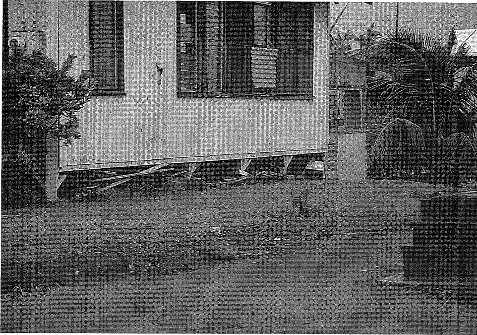
Figure 91. Wood pier foundation shifts under the shear forces created by the wind.
