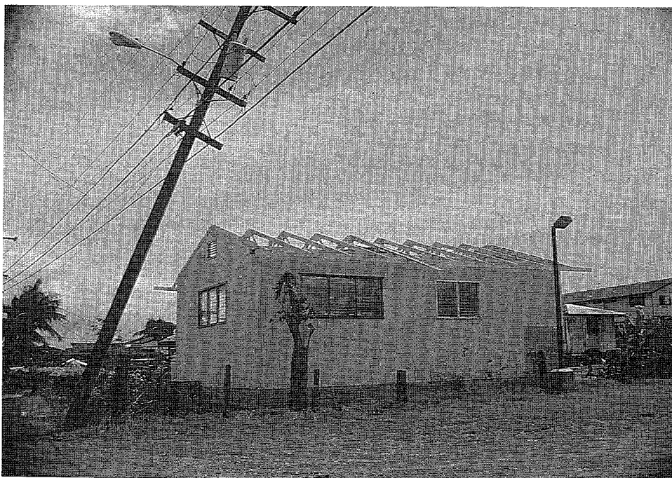
Figure 78. Roof purlins stripped from roof along with metal roofing. Purlins were commonly fastened to trusses with only one nail at each intersection.
