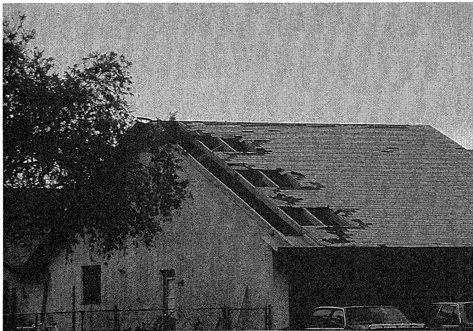
Figure 24. Illustration of wind damage to rake overhangs when overhang framing was not anchored back into the roof system.
