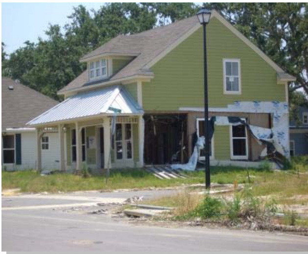
Exhibit 2-8. Property in “Poor” Condition
