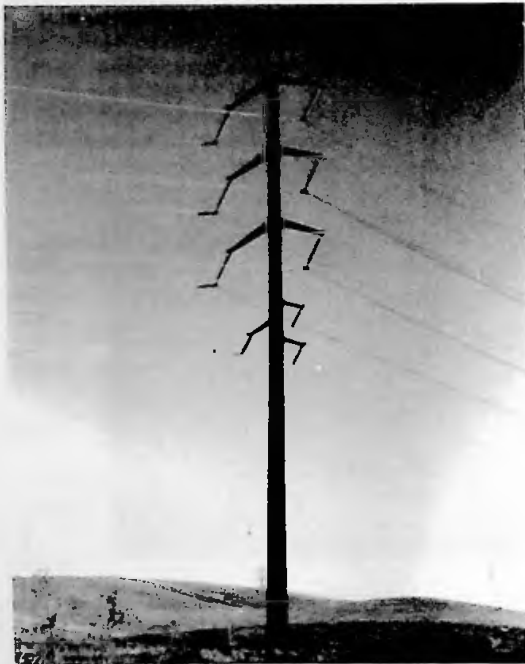
Figure 6-2 230-KV Double Circuit Transmission Line With 115-KV Underbuild Transmission Line on Steel Pole
