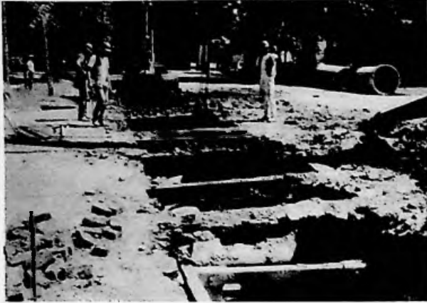
Figure 5-1 Pipe Removal and Replacement is Complicated by Utilities, Railroads and Other Surface and Subsurface Features. Courtesy, City of Sacramento, California
