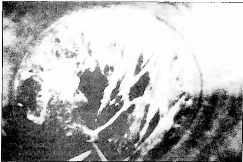
Figure 3-13 Serious Root Intrusion. Courtesy Rodding-Cleaning Services, Inc.
