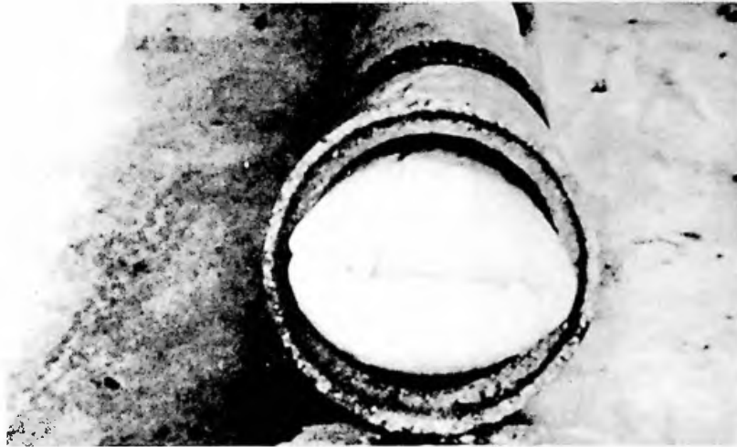
Figure 5-36 End of the Resin - Impregnated Liner During Inversion. Courtesy of Insituform of North America, Inc.
