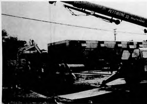
Figure 5-2 Removal and Replacement of Large Diameter Pipes Requires Major Disruption of Streets. Courtesy, City of Sacramento, California
