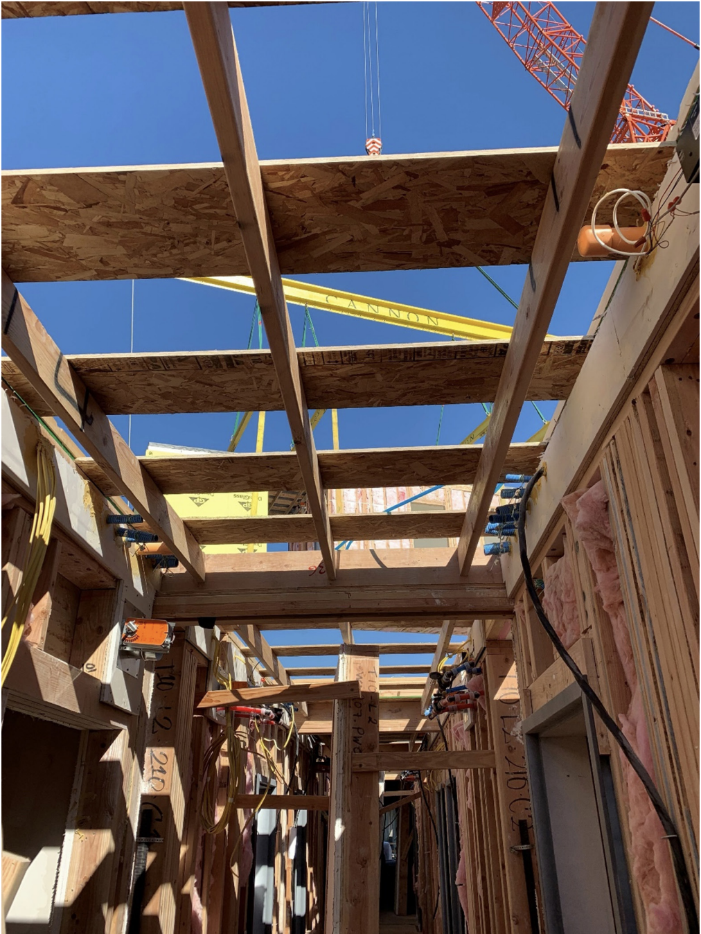
Hallway photo showing site-built connections planned for corridors. Image courtesy of Factory_OS.
