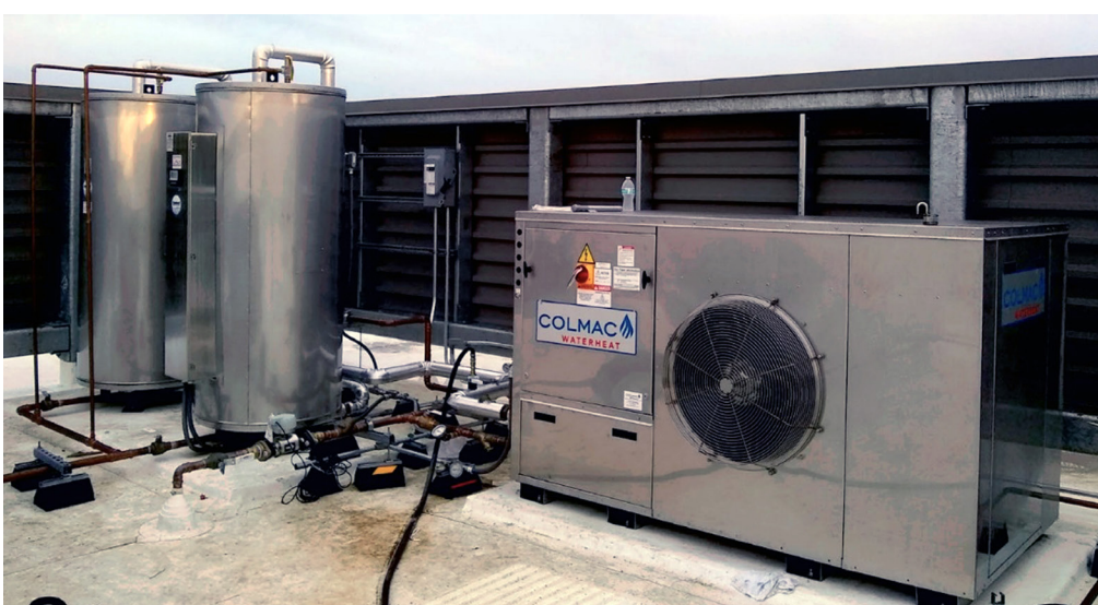
Large installations on roof are most common. Used with permission of Colmac WaterHeat.
