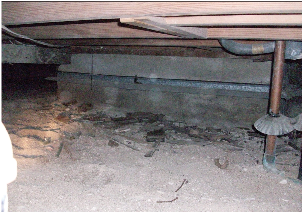
Crawl Space Under a Conditioned Living Area With Missing Floor Insulation
