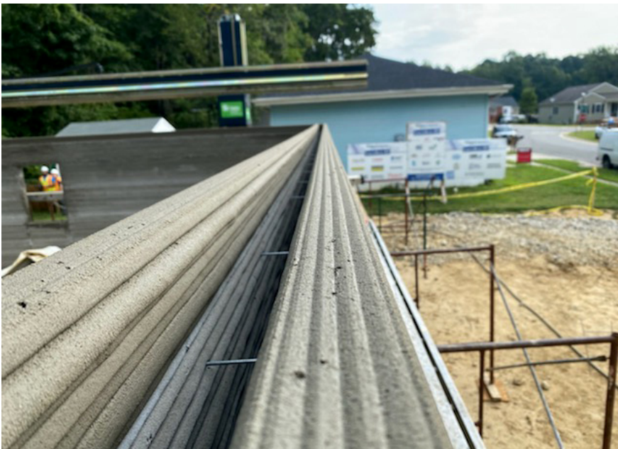
Top view of newly printed wall with metal frame for robotic gantry-arm in the background.
