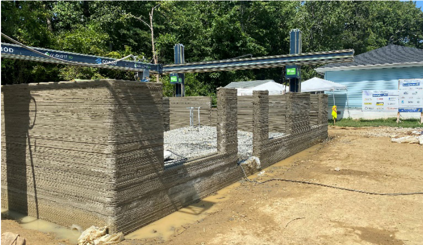
Layered walls that make up the outer frame of a home being built with 3D concrete printing construction.
