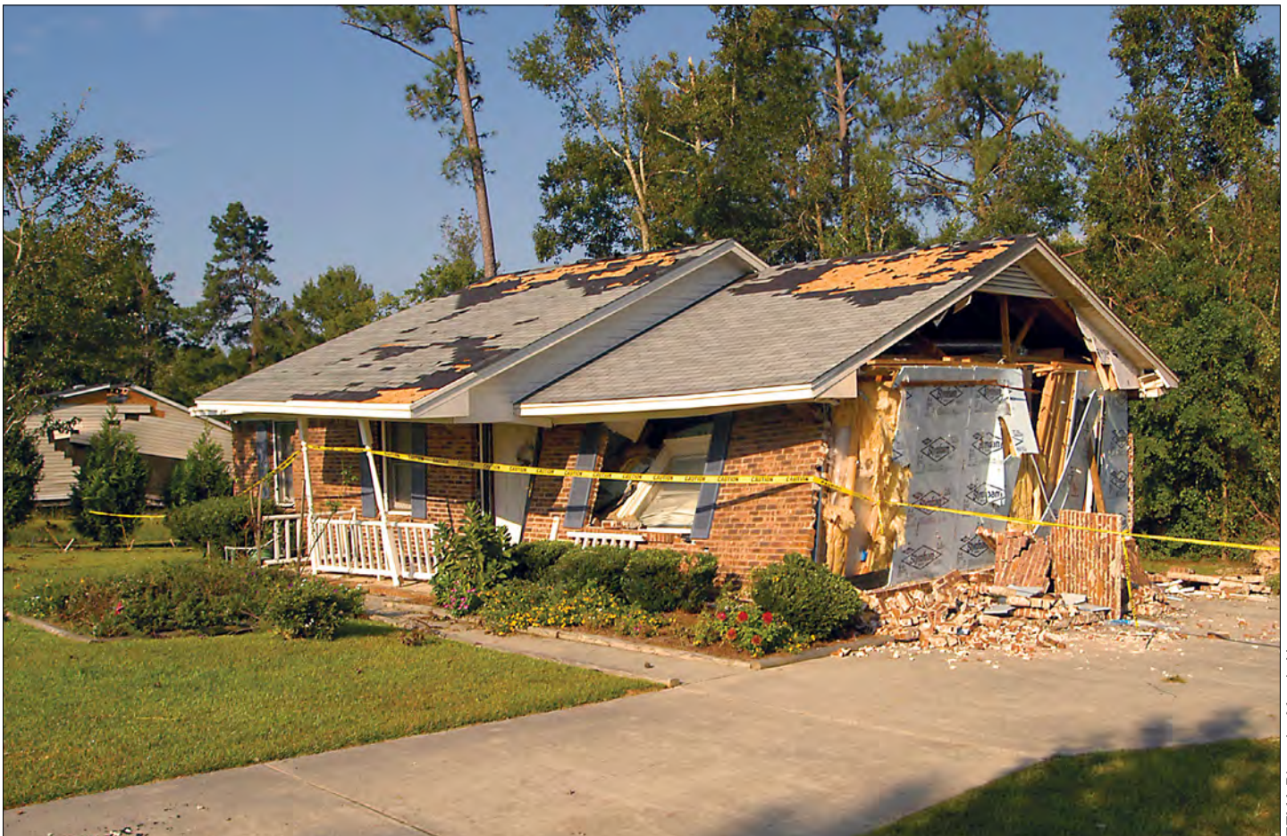
A home severely damaged by high winds in Sumter County, South Carolina.
