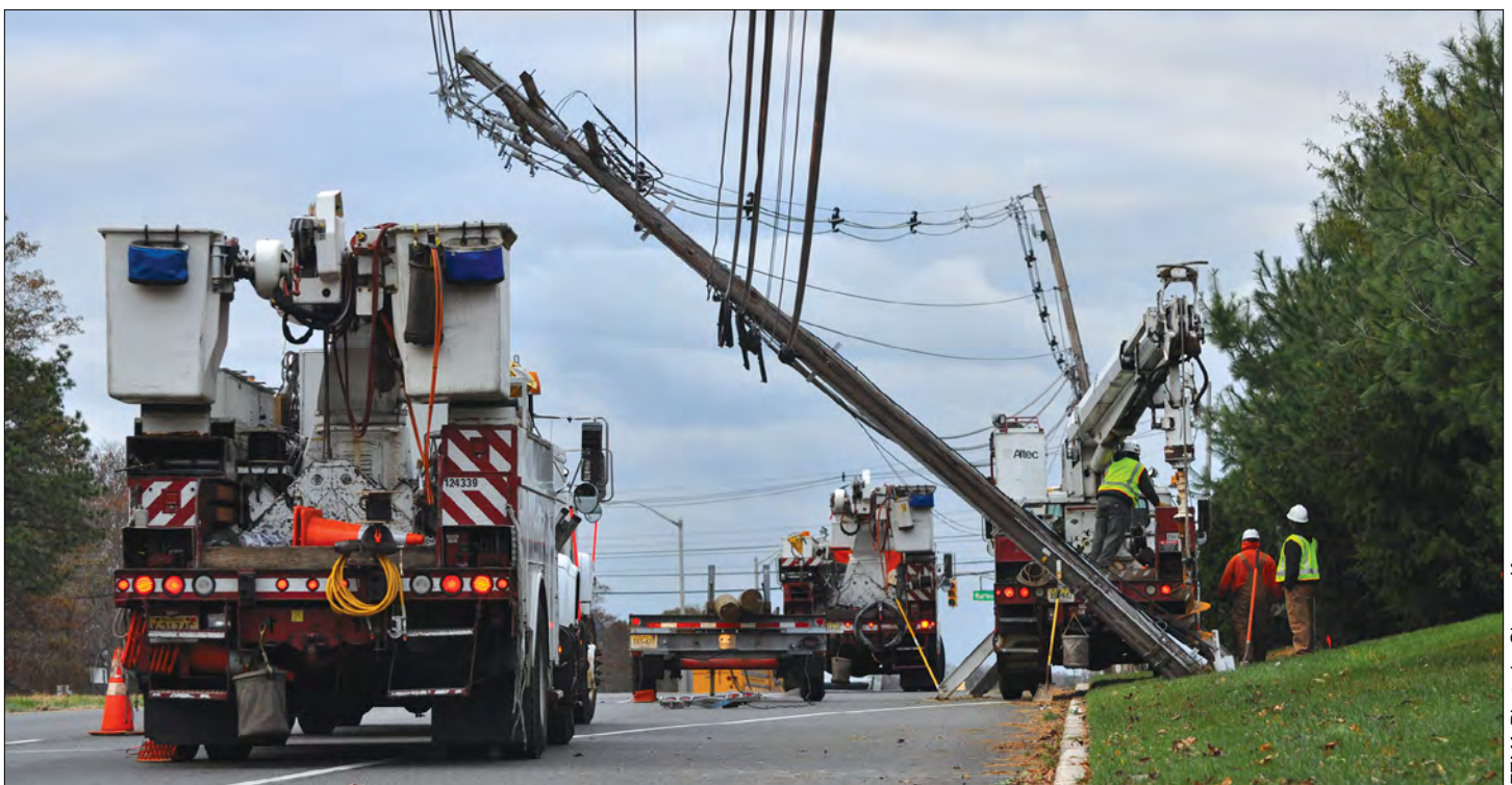
Crews work to restore electricity in New Jersey following Superstorm Sandy, which caused outages for more than 8.5 million customers.
