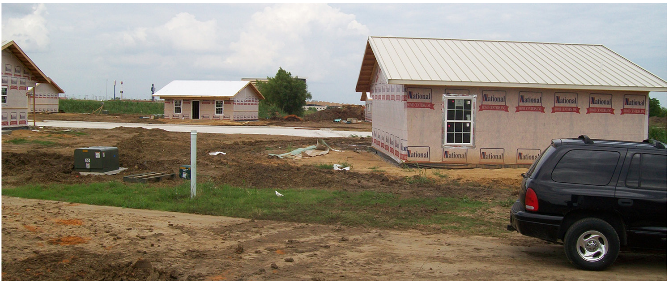
Homes being built by the Choctaw Nation in Durant, Oklahoma using green building standards and funded by the American Recovery and Reinvestment Act of 2009. Image courtesy Southern Plains Office of Native American Programs staff.
