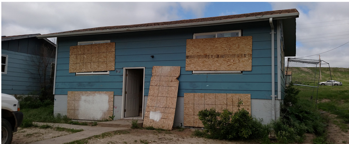
1937 Act house on the Pine Ridge Indian Reservation designated for rehabilitation using Indian Community Development Block Grant funds for mold remediation.
