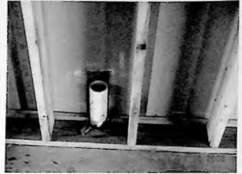
Fig. 3.42 Underslab pipe falls in firewall plan; field modification damages firewall
