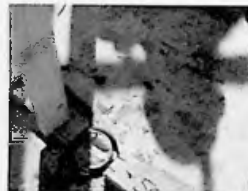
Fig. 3.63 Plumbing misalignment discovered after panel installation (2)
