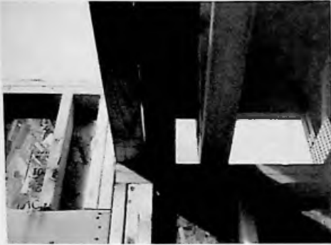
Fig. 3.43 Superintendent's observation of missing truss
