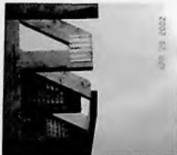
Fig. 3.70 Truss end misalignment and field modification
