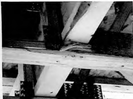
Fig. 3.40 Preengineered component damage
