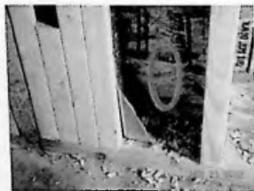
Fig. 3.91 Hurricane tie anchor installed: OSB and tight stud spacing make impact wrench difficult to use
