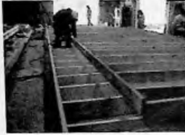
Fig. 3.20 Overall view of roof rafter folded down on ceiling joist
