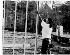
Fig. 3.84 Installing OSB spacers to make up for differences between panels and foundation
