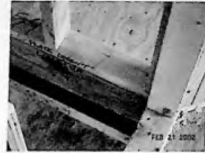
Fig. 3.93 Panel misalignment at stair opening
