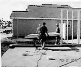
Fig. 3.76 Step 2: With panel positioned, anchor bolt locations are scribed to bottom plate
