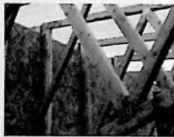
Fig. 3.69 Truss top chord misalignment and field modification
