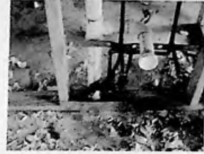
Fig. 3.92 Panel rough-in conflict
