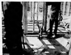
Fig. 3.62 Plumbing misalignment discovered after panel installation (1)
