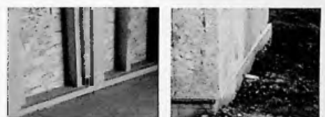
Fig. 3.38 Wall panels and out-of-square foundation
