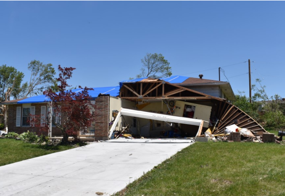
Broken garage door from wind-borne debris.
