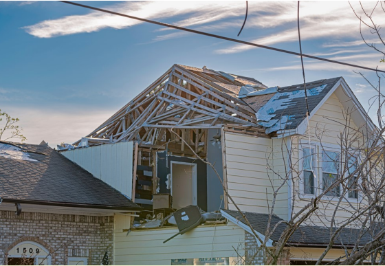
Structure failure due to wind pressurization.
