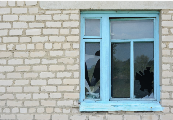
Broken window from wind-borne debris.
