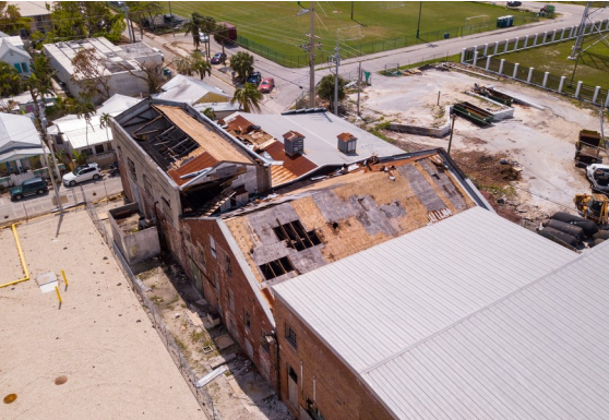
Roof deck, cover, & underlayment damage.
