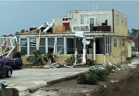
Failure due to lack of load path. Source: FEMA
