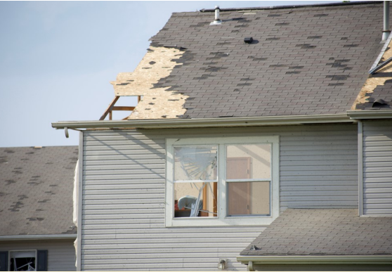
Roof deck, cover, and underlayment damage.
