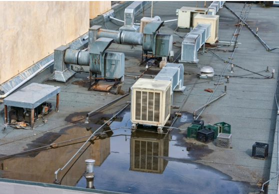
Damaged HVAC unit.
