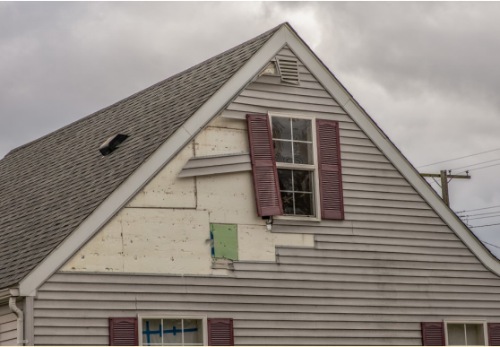
Exterior wall damage from high winds.
