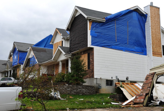
Chimney and wall damage due to high winds.
