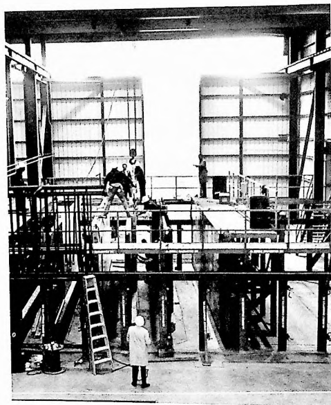
F. Heated battery, vibrated by compressed air. Ten wall panels are poured at one time and removed in three hours.
