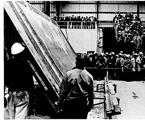
D. Table with finished floor slab tilted to upright position for slab removal.
