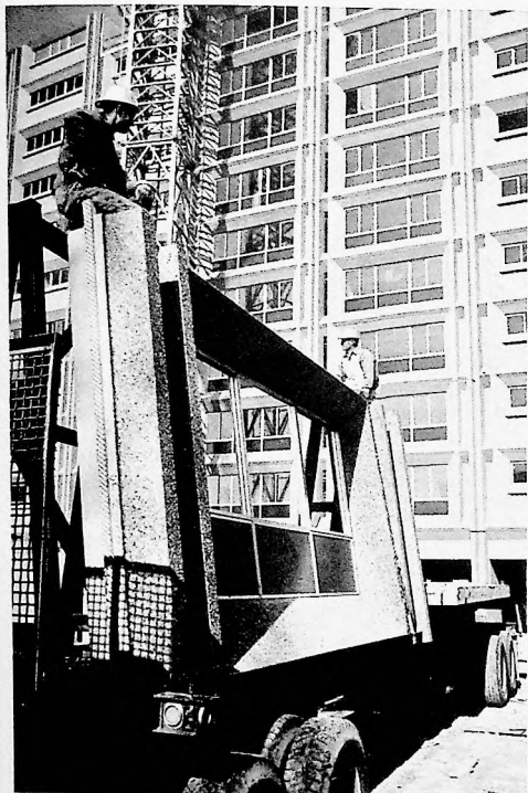
I. Exterior facade panel, with window frame and HVAC grill, ready for installation
