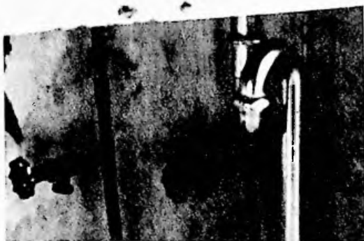
A S-trap that can cause self-siphonage and loss of the water seal. All such traps should be replaced.
