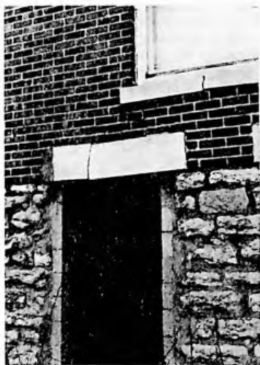
Failure of a concrete lintel and sill due to differential settlement of the building. Permanent repairs will be quite expensive. Note the makeshift shoring of the lintel.
