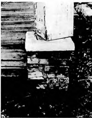
This pier has been overstressed by movement of the porch and column. The entire assembly should be rebuilt.
