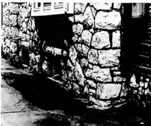
Poor site drainage leads to a variety of problems, in this case a wet basement.
