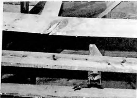
This split ceiling joist can be easily repaired by propping it back in place and bolting new structural pieces to each side.
