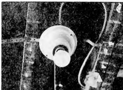
The armored cable and junction box are in good condition and can be reused, even if the lighting fixture is relocated.
