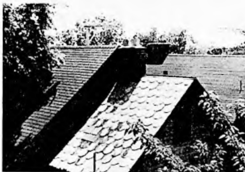
This slate roof should be carefully investigated since it has a makeshift repair. Other problems include the chimney, which is too low, and the vent pipe, which is too narrow.
