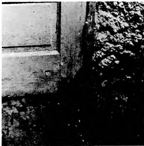
A common location of fungal and insect infestation is where wood door frames touch concrete or earth at grade.
